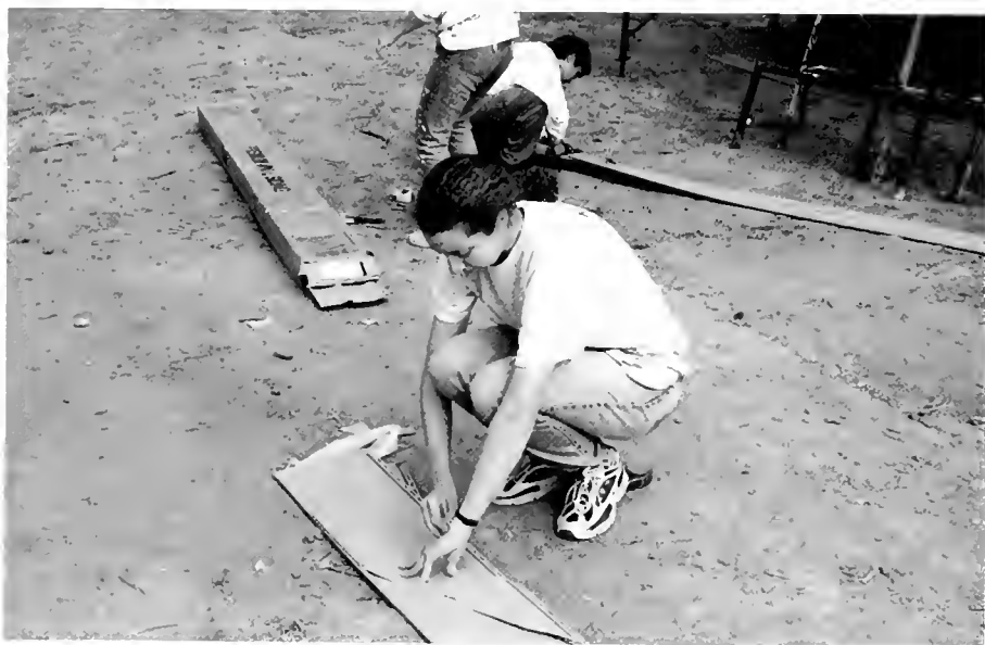
Measuring Up ... Meda Tilghman measures siding for a house in Winston-Salem. Habitat for Humanity builds houses for needy families across the country. (Photo by Robert Numbers)
